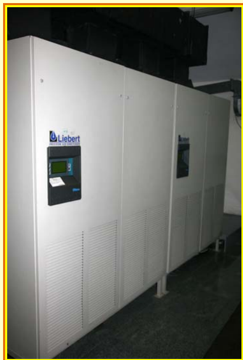
Liebert 8 Ton Air and Humidity control units
